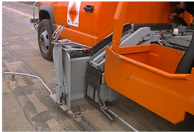
Figure 2-16 Drop box system (Left side)
