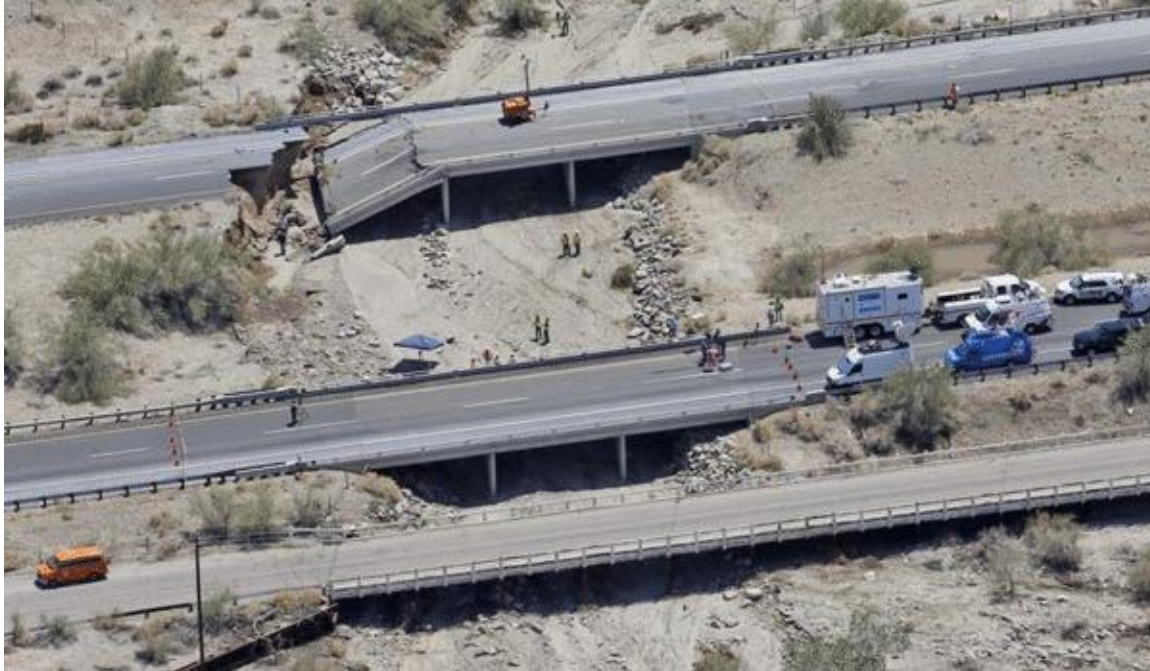
Figure B.3: Caltrans SATCOM trailer emergency use at an I-10 bridge collapse
