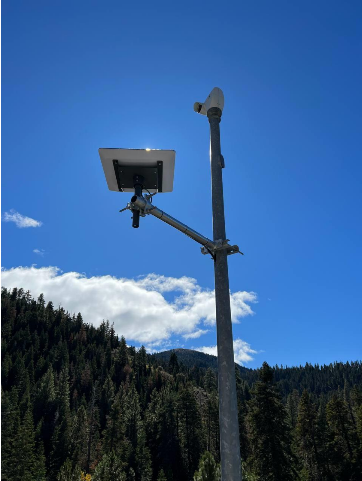
Figure 2.15: First view of a complete Starlink Ground Pole installation at a field site
